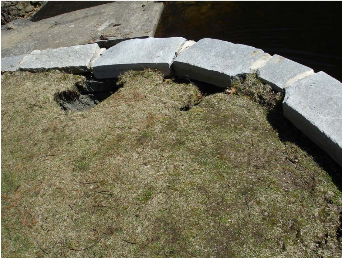
Photo 3 – Sinkholes on left embankment looking toward the spillway
