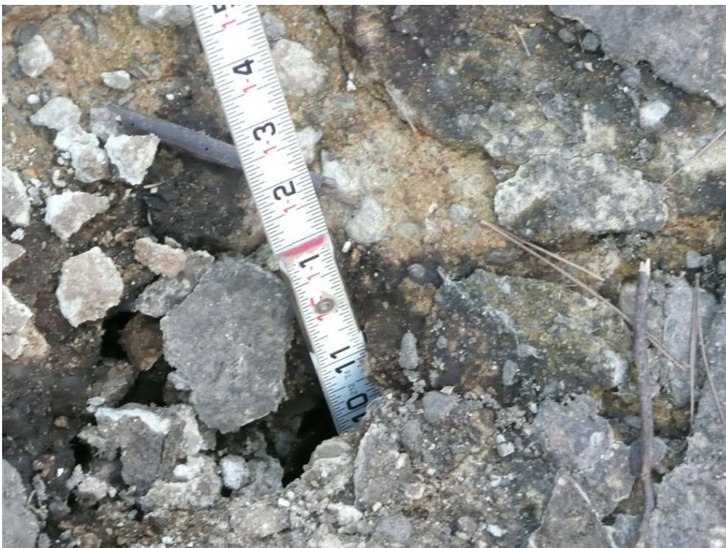
Photo 8 – Spillway crest void*
