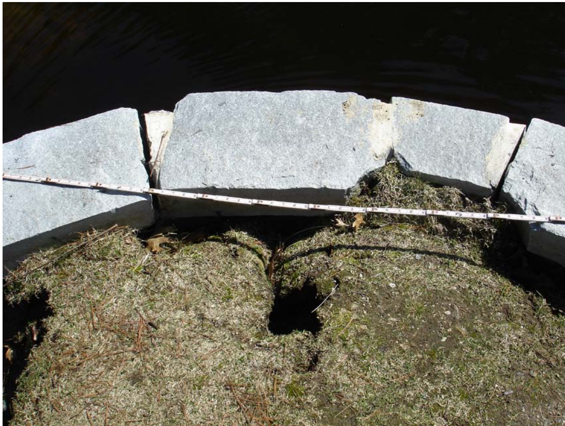
Photo 5 – Left spillway wall, cracked joints, and sinkholes
