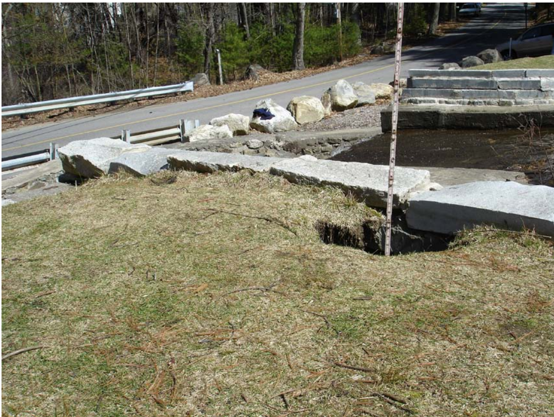
Photo 4 – Sinkhole on left embankment looking toward the spillway
