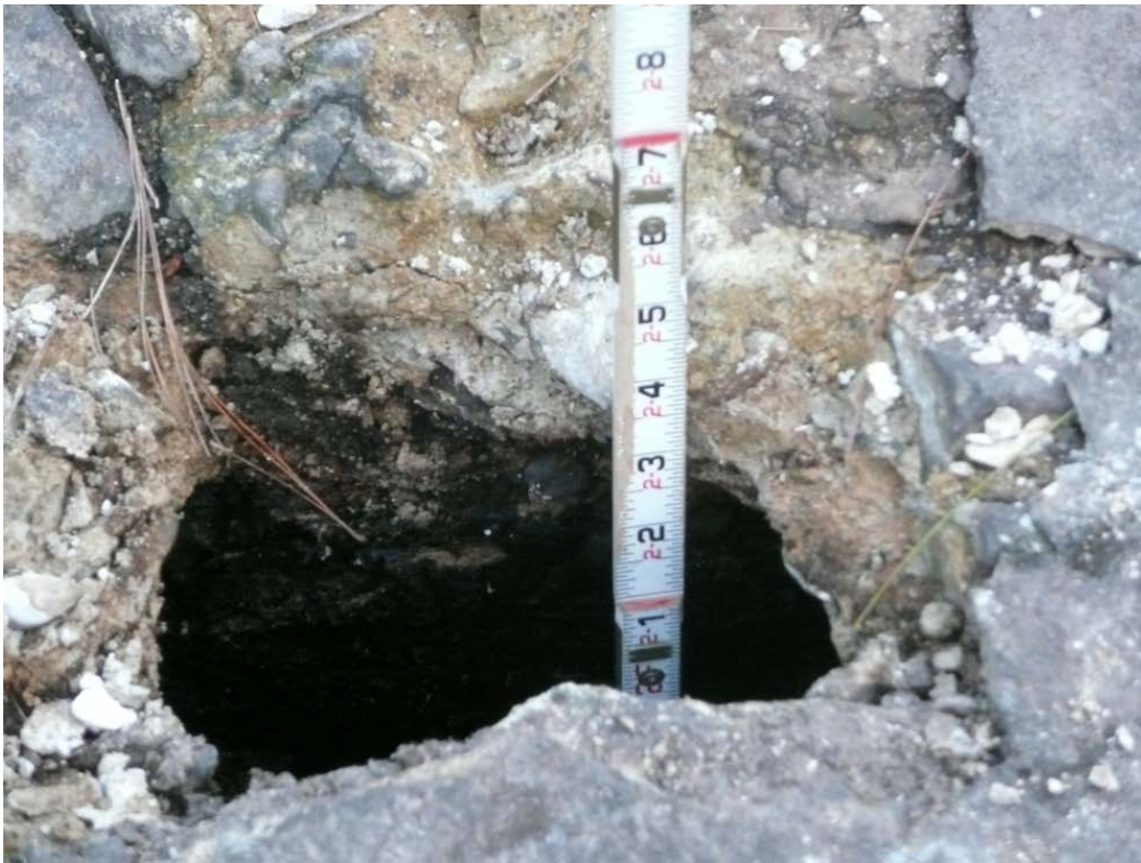
Photo 7 – Spillway crest void*
