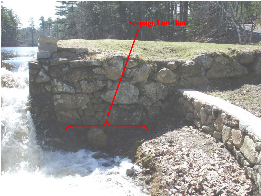
Photo 1 – Seepage locations along left downstream wall from downstream
