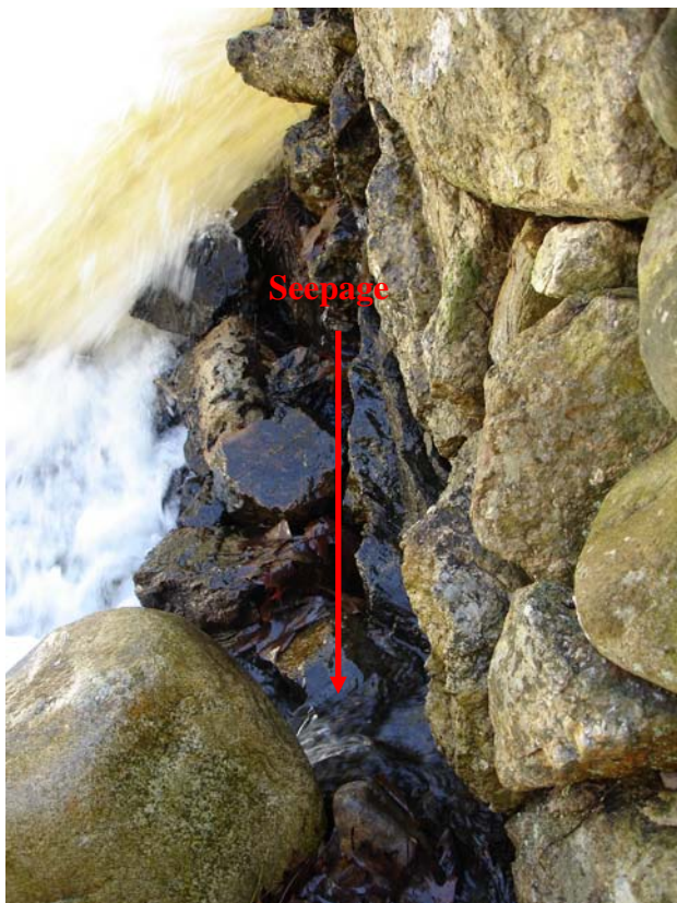
Photo 2 – Seepage, looking down at wall base
